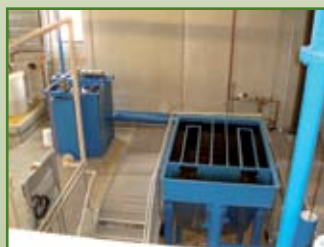
Photo from top of plate settler where backwash sludge is being settled/thickened
