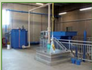
New reclaim system (plate settler and polymer feed system)
