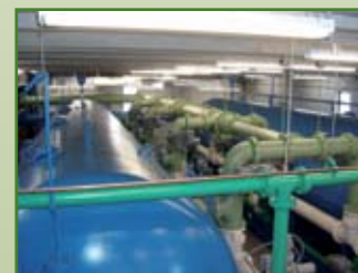
New filter room / piping (from catwalk above)
